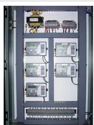
A metering box for a district heating system.
