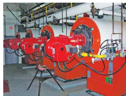
The boilers that provide heat for North Vancouver's district heating system are serviced and maintained by Corix Utilities.
