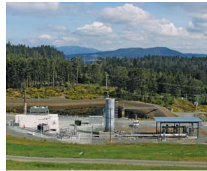
The Hartland Landfill Gas Utilization Project, a partnership of the Capital Regional District and Maxim Power, produces 1.6 MW of green power and returns a royalty of $200,000 annually to the CRD. Source: Capital Regional District
