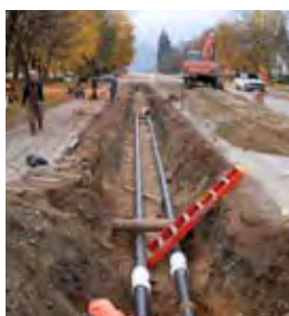
Laying of insulated district heating pipes in Revelstoke. Source: Revelstoke Community Energy Corporation
