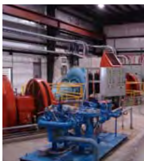
China Creek power plant. Source: Upnit Power Corporation
