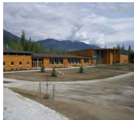
Laying of horizontal geo-exchange loops at LEED™-Gold Crawford Bay Elementary-Secondary School , Crawford Bay, BC; and finished school. Source: Adam James, Community Energy Association
