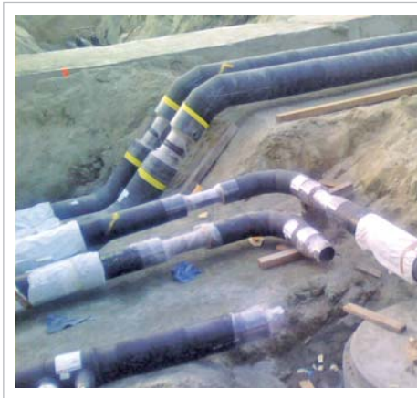
Laying of insulated district energy pipes for the South East False Creek Neighbourhood Energy Utility. The pipes will transmit water, warmed by heat recovered from wastewater, to heat the neighbourhood. Source: Community Energy Association
