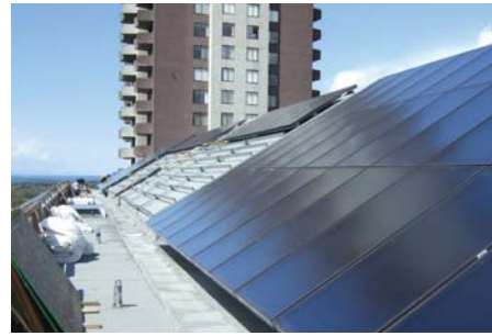
Solar hot water panels under construction on the roof of the City of North Vancouver public library. Source: City of North Vancouver
