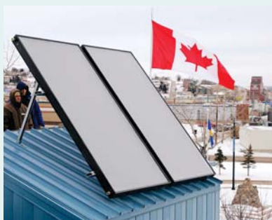
Solar panels heating domestic hot water, on the Dawson Creek City Hall. Photo source: City of Dawson Creek
