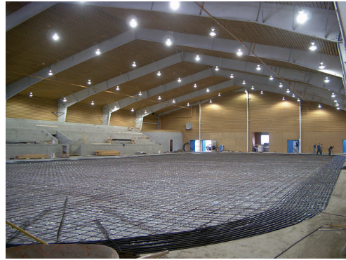
South Cariboo Recreation Centre ice rink: Ground-source loops before the concrete is poured; these loops cool the ice. Additional loops under the concrete heat the ground to prevent permafrost.
