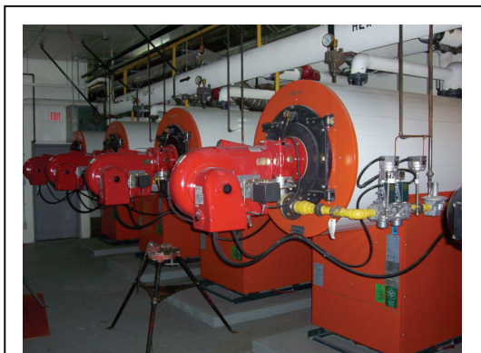
Boilers to heat the hot water for North Vancouver's district heating system are located in a small area of a parking garage. Source: Community Energy Association
