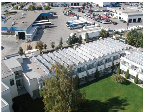
102 solar panels and heat recovery system, heating water for the hotel, on the roof of the Best Western Inn, Kelowna. In addition to solar technology, the system recovers waste heat from the hotel's air conditioner to help heat the water in summer.
