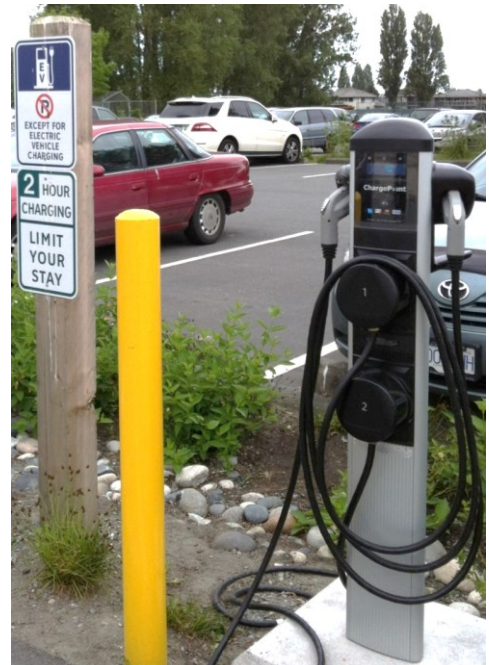
Commercial Level 2 Charging Equipment
