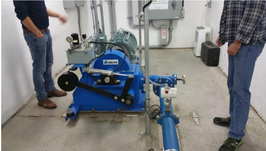
Figure 9 Nakusp Micro Hydro System
